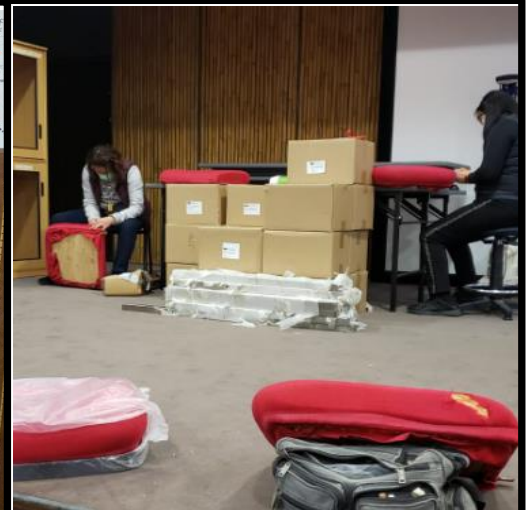
We have repaired total 7 nos of seat rests with fabric problem, now can use as normal.
