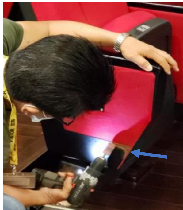
7A) Technical staff is fine turning the 生鏽 corner, remove 生鏽, cleaning preparation work before painting. (Change to new 不銹鋼 screws)
